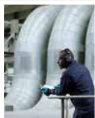
Ruggedised hand and hearing protection, like the Honeywell designed ones shown on this month's front cover, are a requirement at noisy locations such as this power station, where massive pipes collect and transport steam under high pressure. See page 16.
