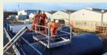
Setting up equipment on tank top in preparation for Internal tank cleaning operations
