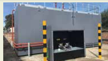
Installation carried out at a depot in Sandwich. Works included decommissioning and removal of the old tanks and demolish brick piers. Then Installation of new banded tank, pipework and header box.
