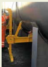
Tank jacking operation to aid the installation of compensation plates following an internal inspection
