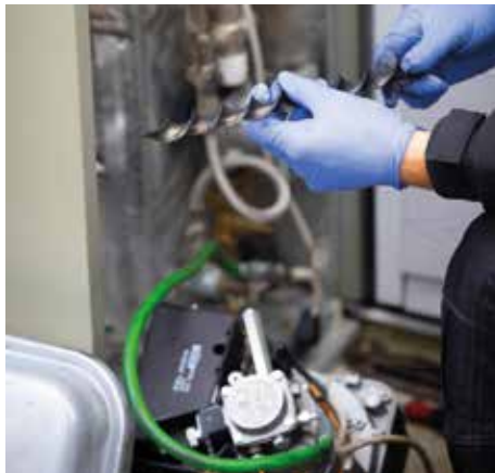
Pictures 12months on showing how clean the internal boiler baffles are, running on HVO
