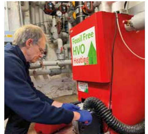
New Boiler at Gwinear School. Trials on their previous boiler so successful they invested for the future with a new boiler
