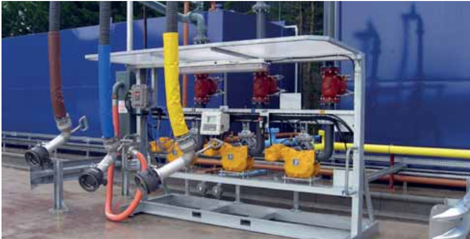
An IFC Inflow system at the Carrs Billington depot in Carlisle
