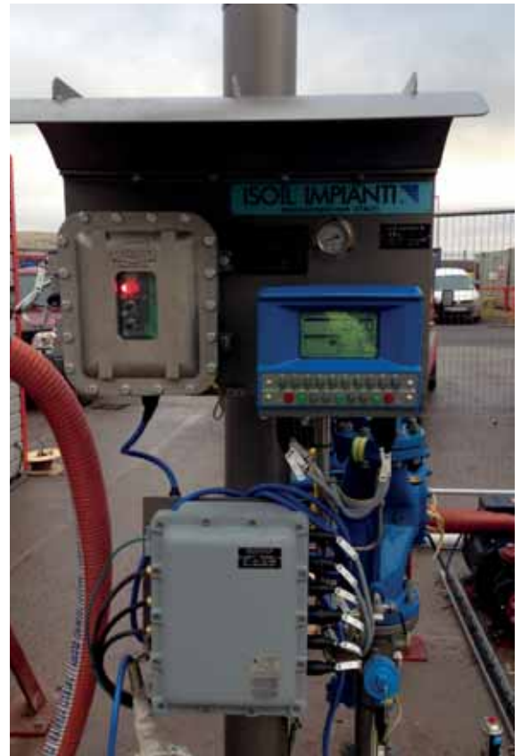
Liquip – a 4" single arm metering system on the Shetlands
