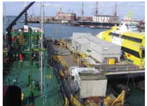
An OTS installation in Portsmouth featuring two fully bunded tanks with dispensing pumps, hose reels and process control equipment
