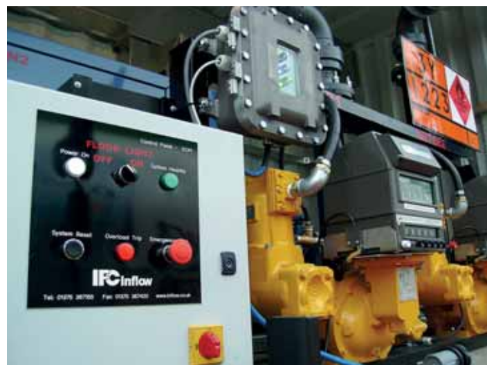
MODSS pumping station
