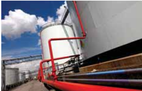
Inter Terminals operates 8 terminals in the UK, Ireland and Germany with a combined bulk liquid storage of 1.23 million m 3 and 4 terminals in Denmark with 1.8 million m 3 . The company handles 250 different products and blends
