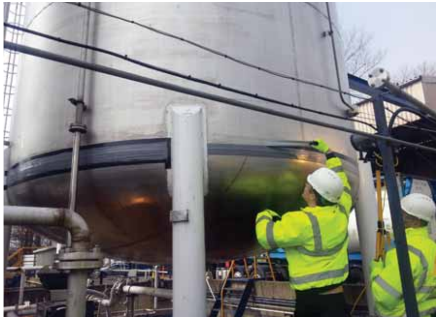
Before – leaking tank After – completed application being unmasked
