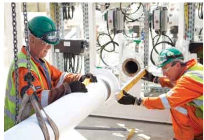
Major investment has been made at import and storage terminals; Greenergy holds its own physical oil at eight terminals, including North Tees shown here
