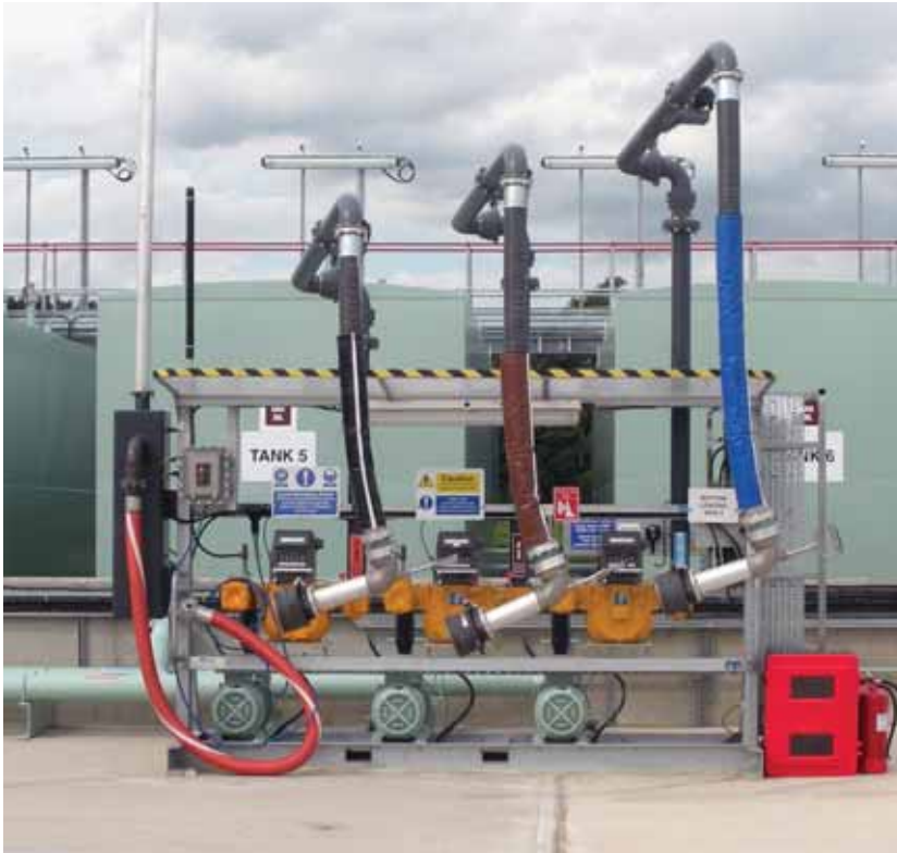
IFC recently installed new equipment at Pace Fuelcare's Ipswich depot
