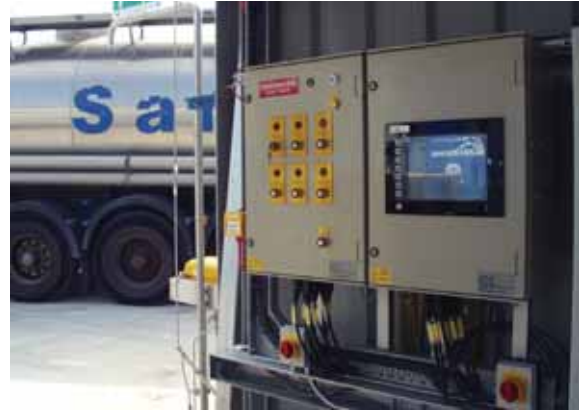
ISS – providing safety and accountability on a chemical site in Wales
